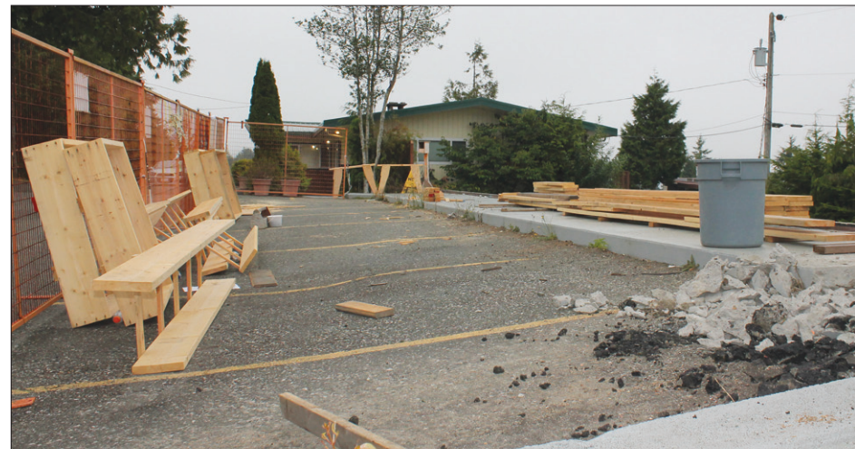
Construction has started on the re-building of the Thornton Motel. The middle block of the motel was destroyed by fire last summer; it should be re-constructed by the spring 2015.
