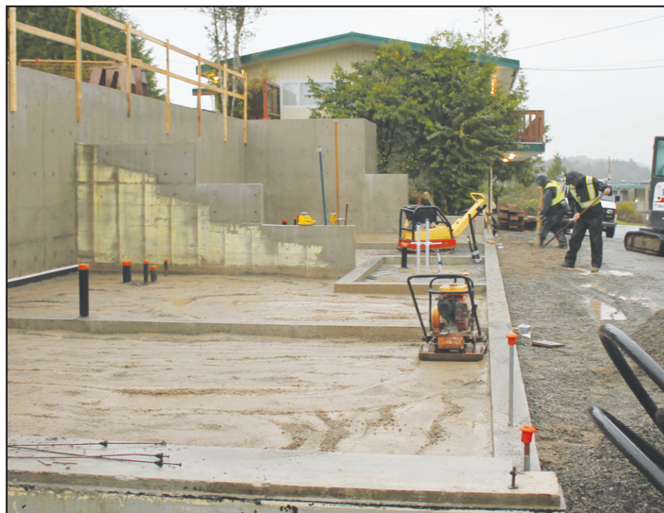
The foundation work has been completed on the re-build of the Thornton Motel and the framing is expected to begin shortly. The motel's centre block was ravaged by fire a year and a half ago. Construction is slated to be completed by the spring.
