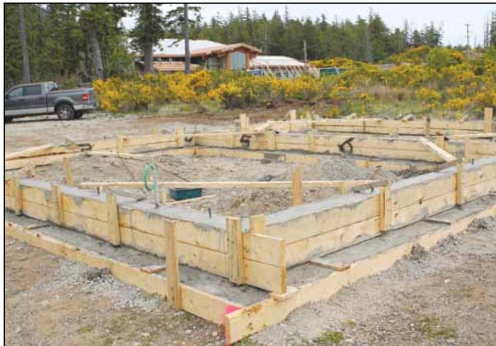
Cement foundations have been poured as the construction of seven new small homes in Hitacu has begun. It is expected the homes will be finished by the end of the year.
