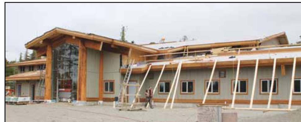
The new Hitacu Community Centre. Sidewalks will be poured in the next couple of weeks.
