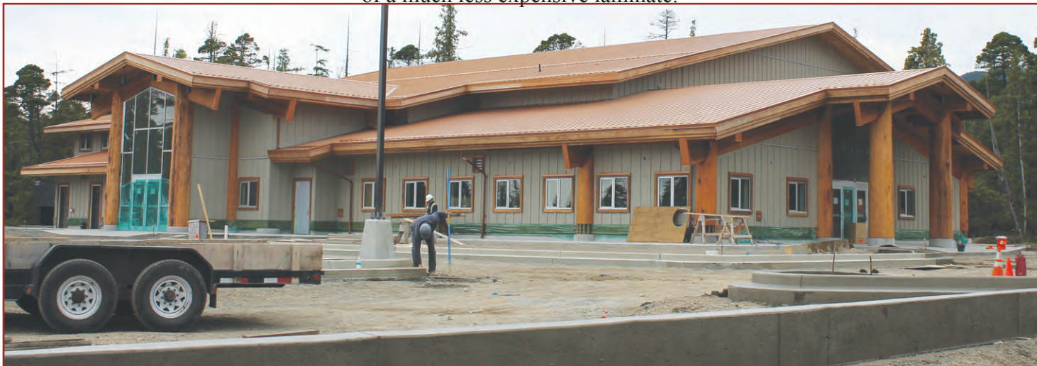
The new community centre has gone about $200,000 over budget and the Executive has decided not to request money from the Settlement Trust to cover the short-fall. Instead, the Executive suggested that items such as landscaping could be scaled back and that a fund-raising effort be launched to cover the short-fall. Construction has been delayed a few weeks and will not likely be completed until mid October.
