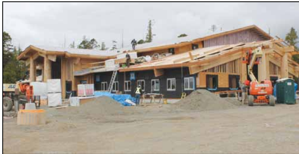
The new community centre in Hitacu is coming along with the roofing now being put on.
