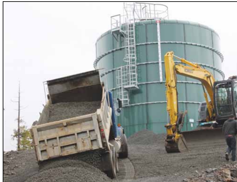
Hitacu's new water reservoir has now been constructed and will go online in a few months once water and sewer upgrades have been completed in the community.
