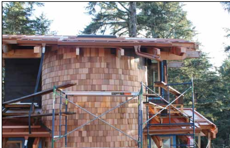
The turret on this lodge boasts a spiral staircase and an amazing bird's eye view of spectacular Wya Beach and beyond. Top photo shows one of the lodges nearing completion.
